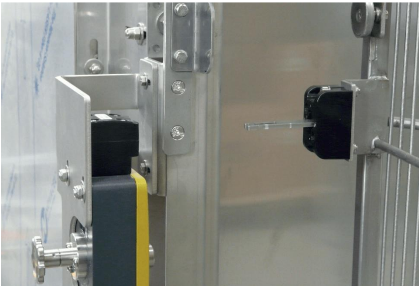
Fig. 3 The safety doors on the Concordia systems are safeguarded by the Ex STM 515.
